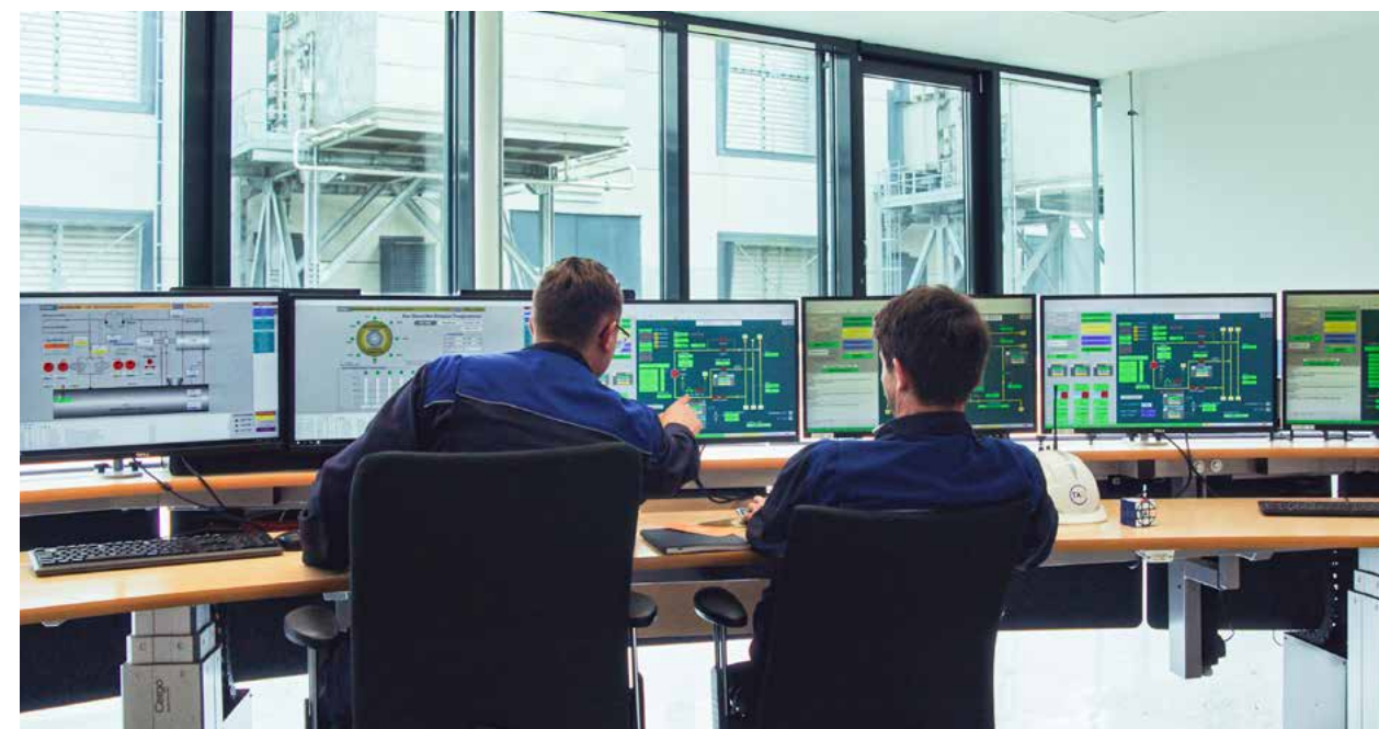
Control room at the Weitendorf compressor station.
